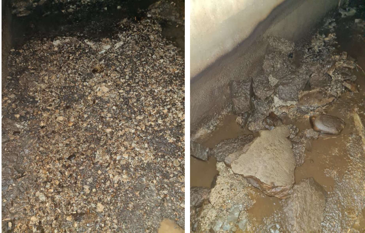
Debris deposited inside the tunnel - pictures N9 and N10
