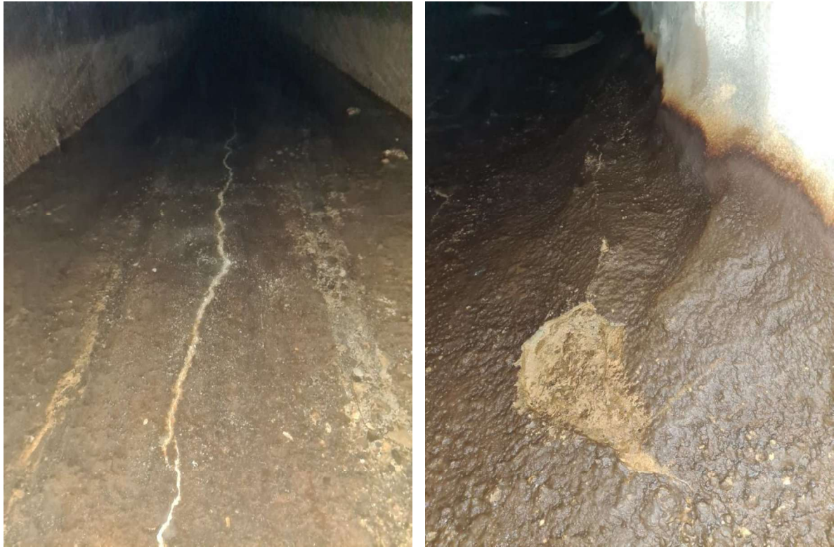
Bulging and damaged bottom of the tunnel - pictures N3 and N4
