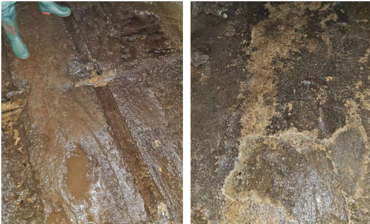
Uneven tunnel bottom - pictures N1 and N2
