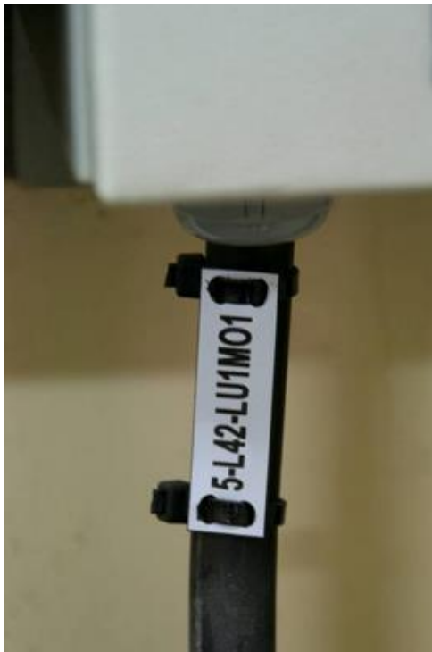
Photo 26: All cables shall be equipped with labels at both ends
