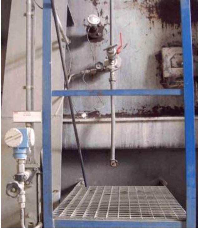
Photo 2: Shows a typical installation of a pressure measurement at the kiln hood
