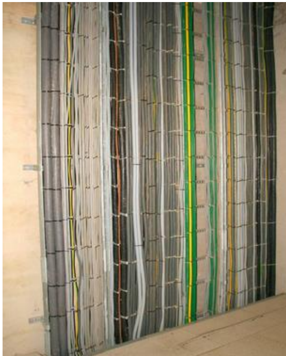
Photo 5: Vertical Cable routing
