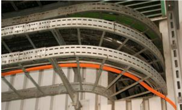
Photo 10: Cable Tray Horizontal bend
