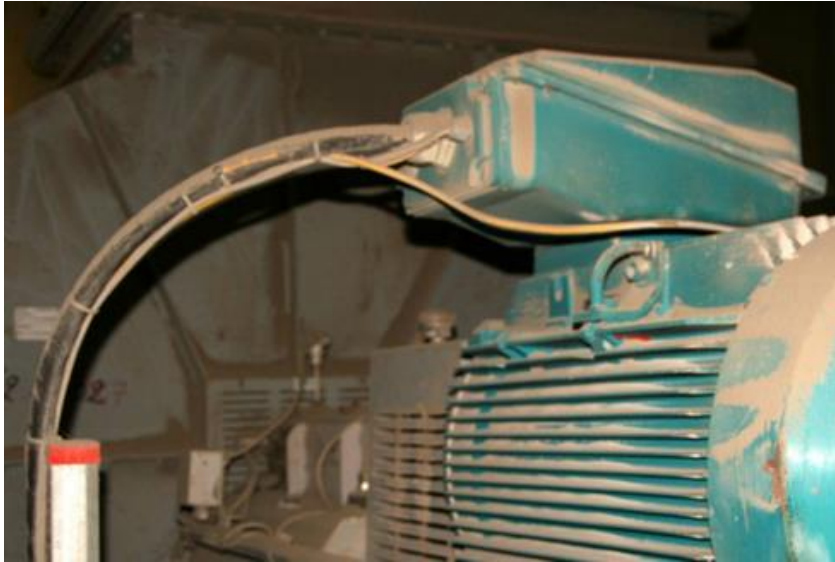
Photo 25: Cable loop is not required on large diameter cable.
