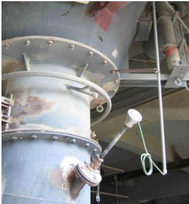
Photo 3: Shows a typical installation of a temperature measurement in the pre-heater
