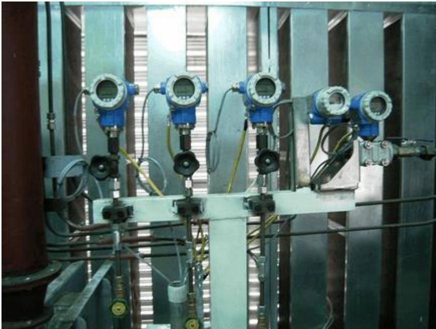
Photo 1: Shows the installation of pressure transducers with valve for shut off and cleaning
