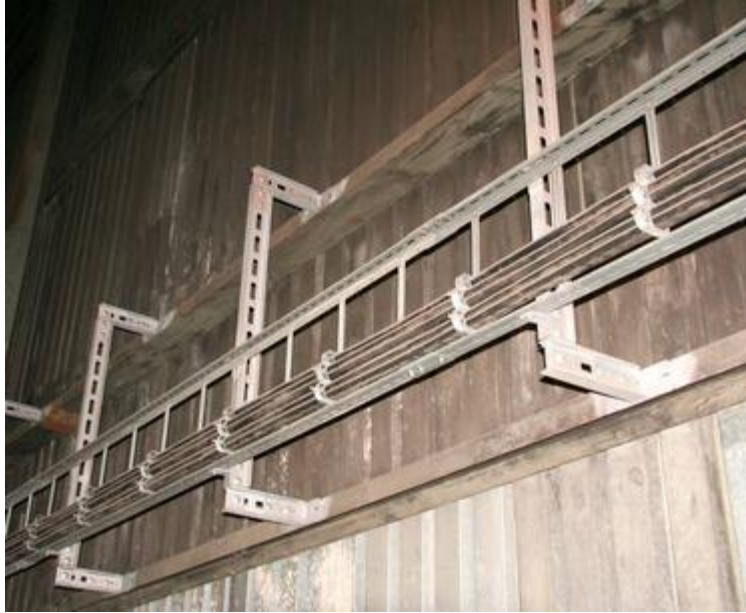
Photo 6: Horizontal Cable routing
