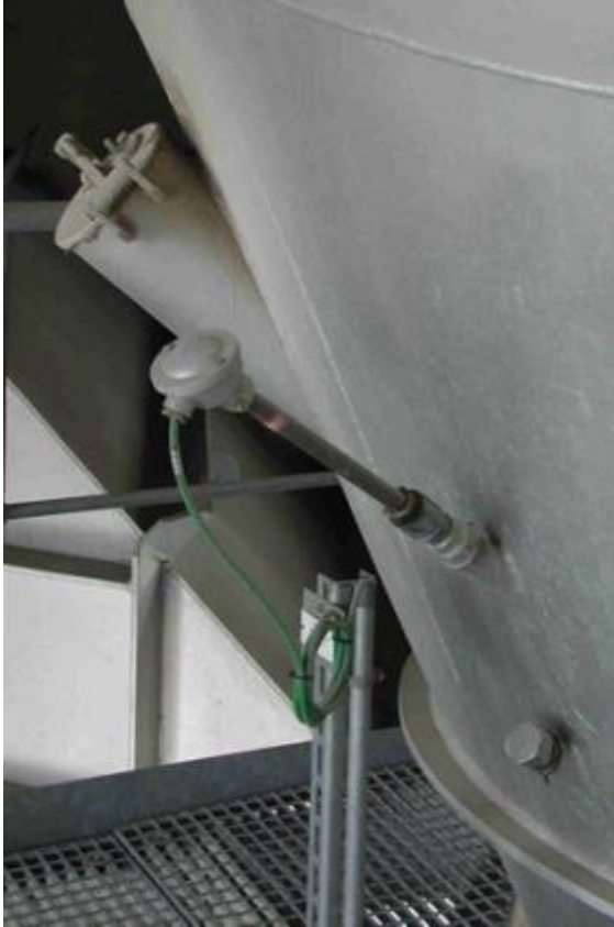
Photo 4: Shows a typical installation of a temperature measurement in the pre-heater
