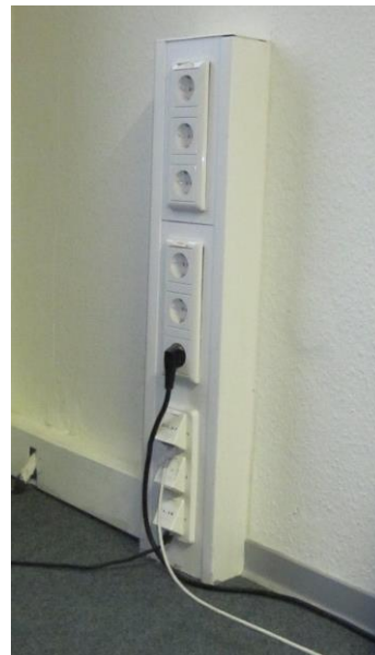
Photo 37: Cable routing in Offices
