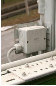
Photo 1: Lighting Junction box
